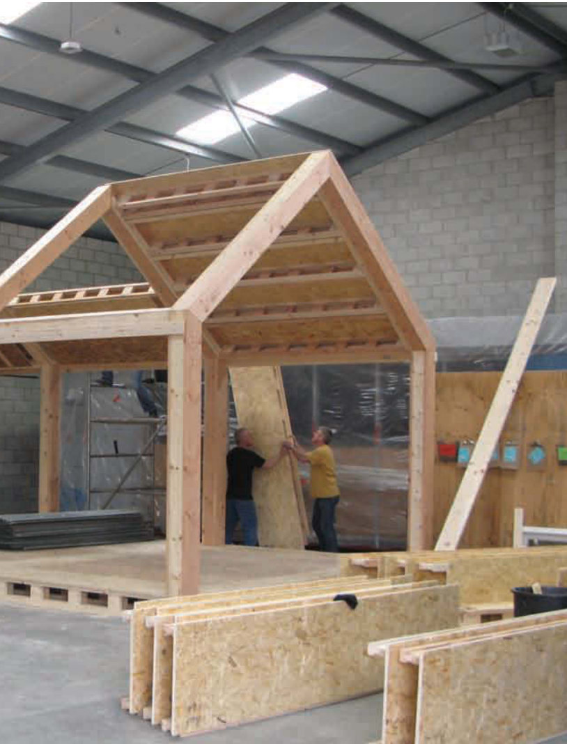
The Ty Unnos system which resulted is a highly adaptable modular system that can create a range of house types and sizes based on four standard modules.
